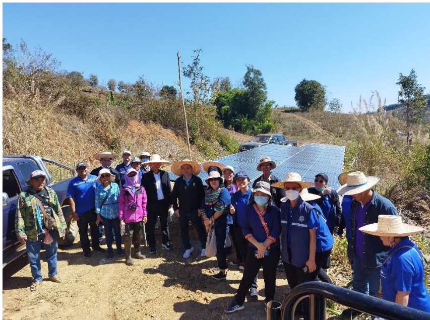
Solar irrigation system at Ban Mai Mongkol (Village 2)
