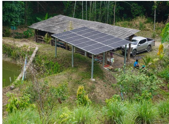
Solar irrigation system at Ban Tabman (Village 4)
