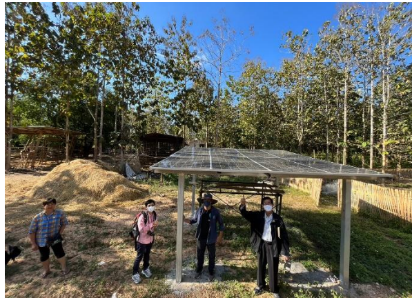
Solar irrigation system at Ban Nong Ha (Village 8)
