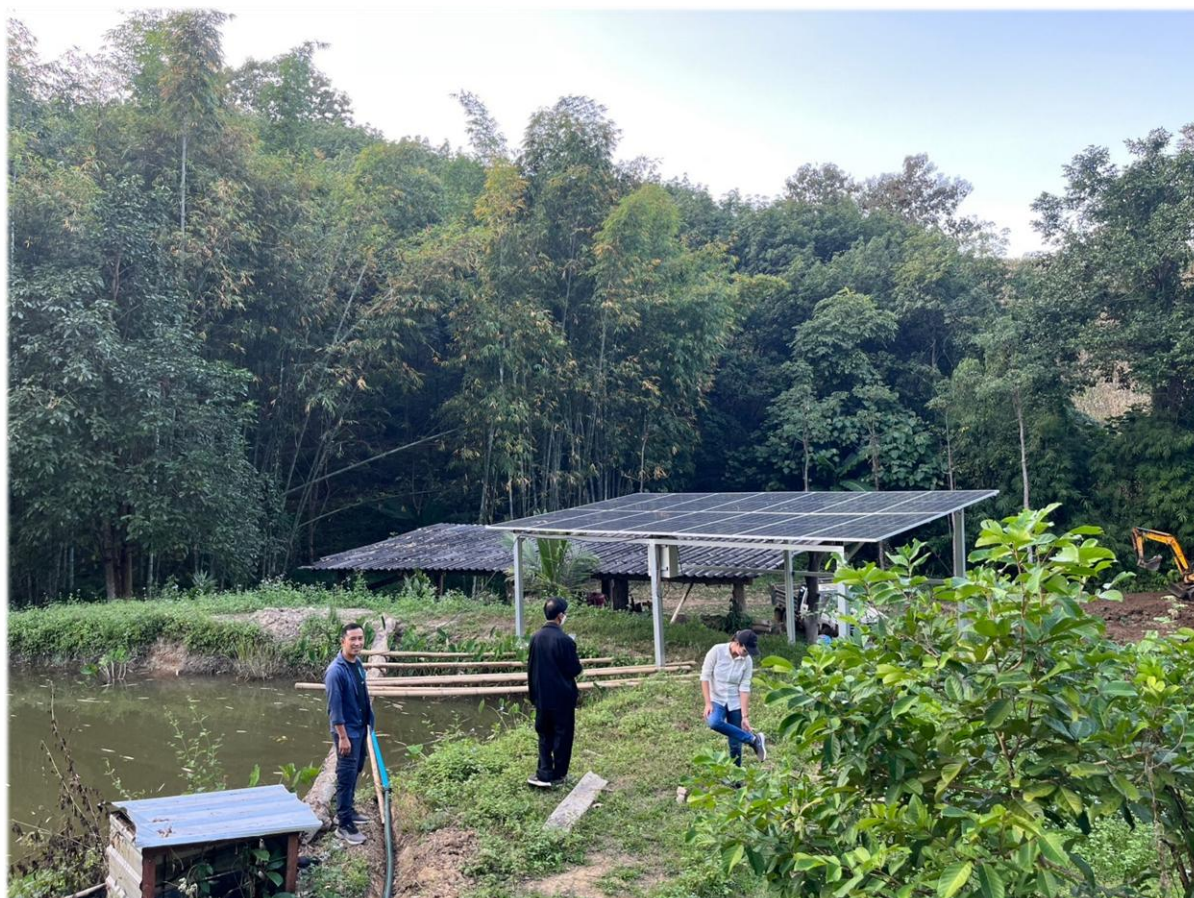
Bua Yai Subdistrict, Na Noi District, Nan Province: Solar-powered irrigation system implementation at the field. Source: Authors.
